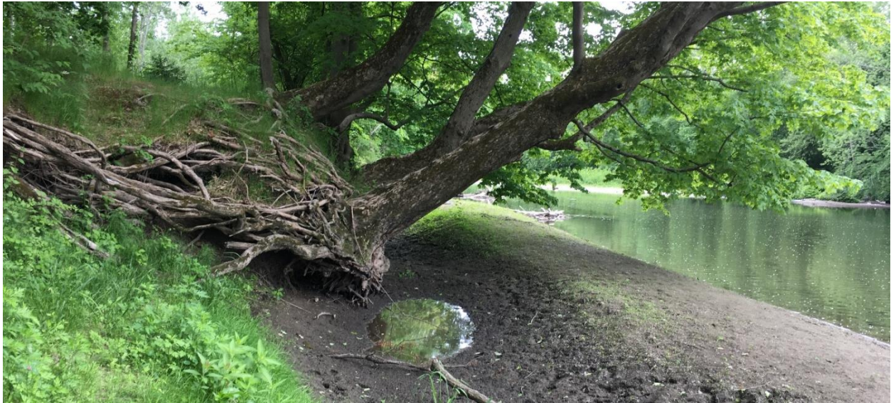
Figure 5: Berming and undercutting of the bank.
