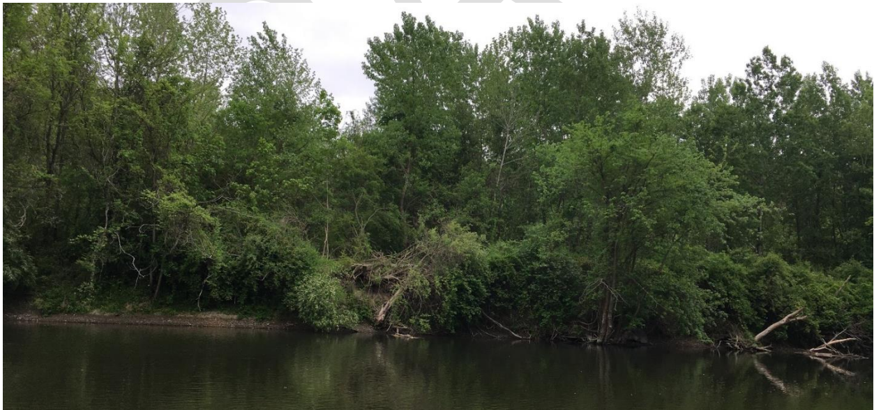
Figure 6: Steep, collapsing shoreline along on the southern side of the Kinderhook Creek.
